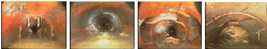
Fig. 5 (a) Hanging Debris (b) Cracked Pipes (c) Grossly Deformed Pipes (d) Blockages
